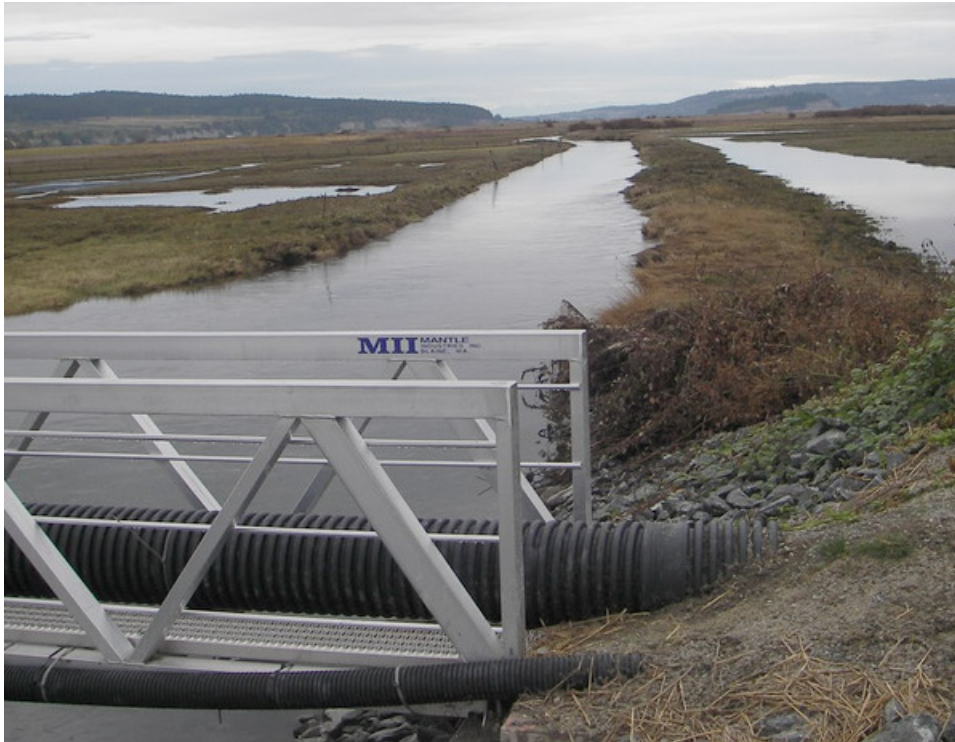
(Pictured left) 9.5 foot trestle for a sewer line crossing at the Crescen Harbor area of the Naval Air Station (NAS) Whidby Island, WA.
